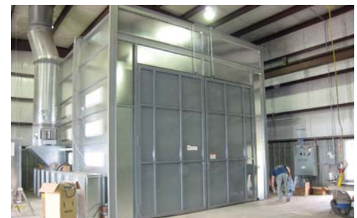
New state-of-the-art temperature controlled paint room
