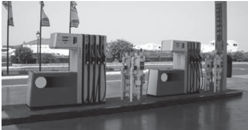
Gas pumps equipped with Vel-Max® Filter Vessels
